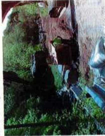
Emergency Watershed Protection Program- Site #501, Beerkill Stream, Town of Wawarsing Ulster County, NY, May 23, 2005. Placement of the rock-construction of the peared rock wall.
