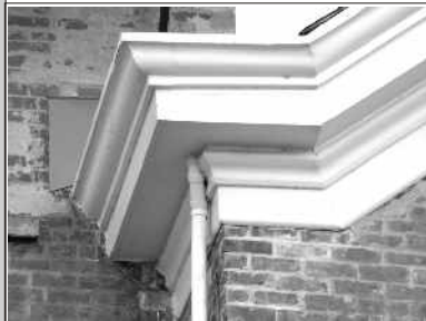
The box cornice that crowns the lighthouse's walls is a typical feature found throughout Saugerties
