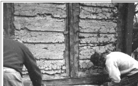
Early Colonial period timber framing insulation method using a clay and grass fiber paste progressively packed between clapboards outside and split sapling lathe inside. The lapped clapboards creates a form that leaves the pattern in the photograph.
